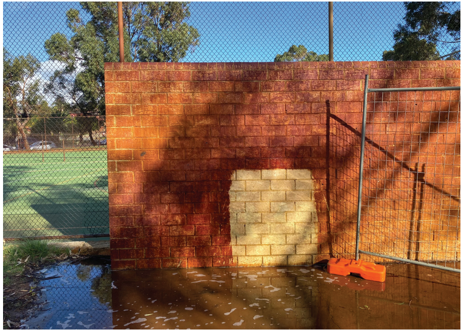
A wall that has been exposed to sprinklers three times a week for several years. Each day, the stain is marginally worse than the day before.
