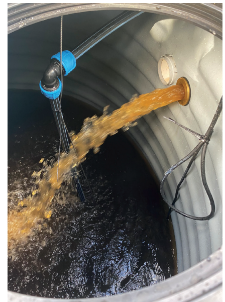
"The goal was to remove iron out of the water and capture it in a separate tank," he adds. "This prevents iron from being used in the school's irrigation," says Oliver
