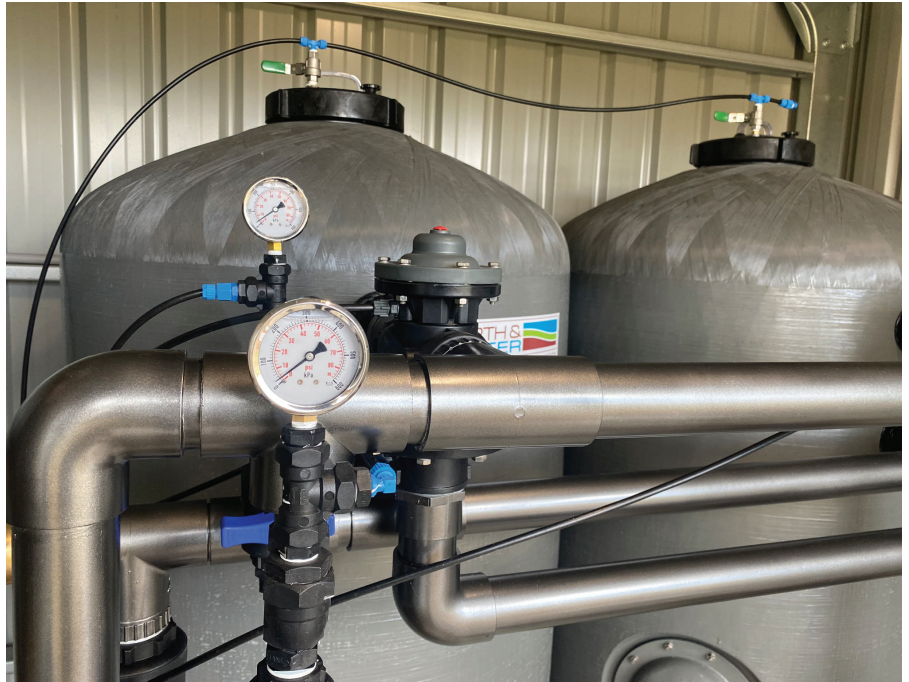
Dual standing Waterco sand filters traps that oxidise and separate the iron from the water.
