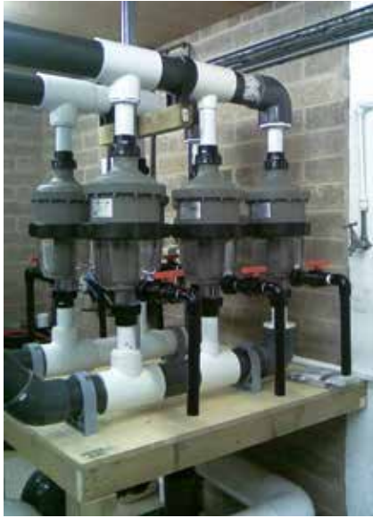
▲ Water is fed through six MultiCyclone pre-filters and then through six Micron Deep Bed media filters filled with glass.
