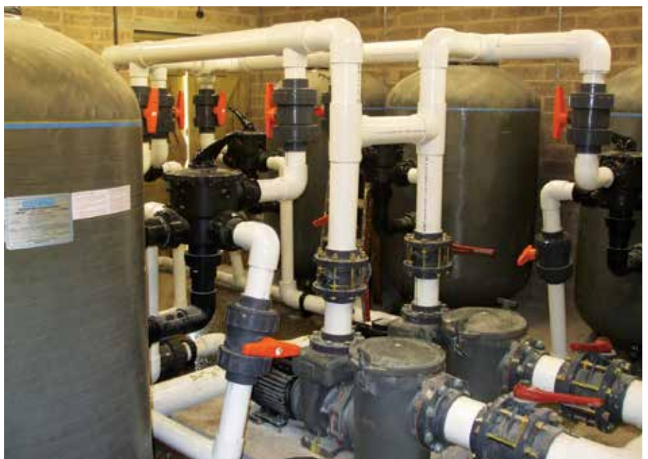
► For the sea lion enclosure, Waterco suggested a chlorinated filtration system using two cast iron pumps connected to existing pipe work.
